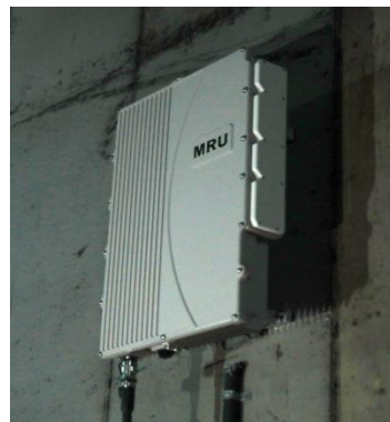
Figure 42 Picture of installed mRU
