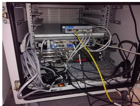
Figure 9 BB Unit assembled in the rack
